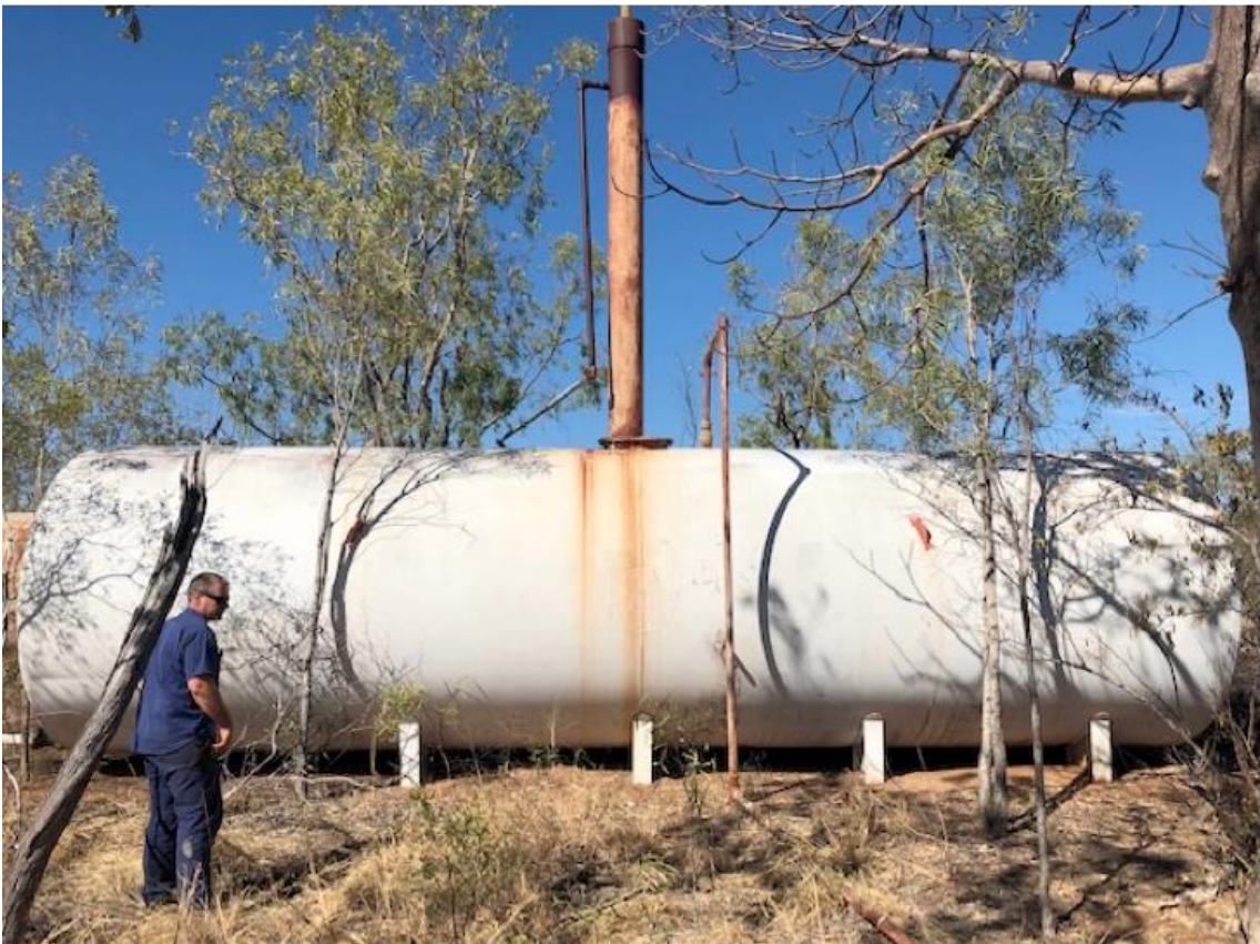
Figure 1: Storage Tanks at West Kora Tank Farm
